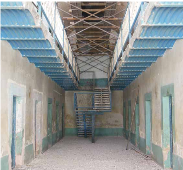
Figure 9. Interior of a pavilion of the outbuilding prior to the intervention. Photograph: Building team of the Leonora
